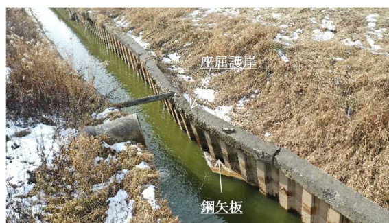
Fig. 1 計測対象の自立式鋼矢板護岸 Steel sheet pile wall to be measured.
